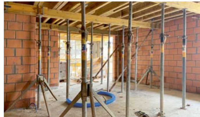
Due to the higher weight of reinforced concrete slabs, many more structural columns are necessary.
