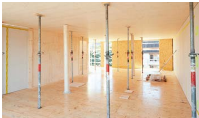
Thanks to minimal temporary support, subsequent trades can start their work even before joint grouting.
